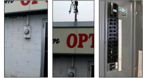
EXISTING SERVICE PHOTOS - LINDSTROM OPTICAL
